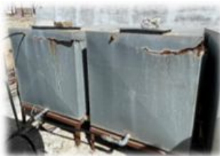
Pictured Left: Old water tanks in need of replacement.
